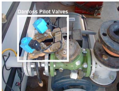
Photo 1. Danfoss Pilot Valves, Lower Bermad
